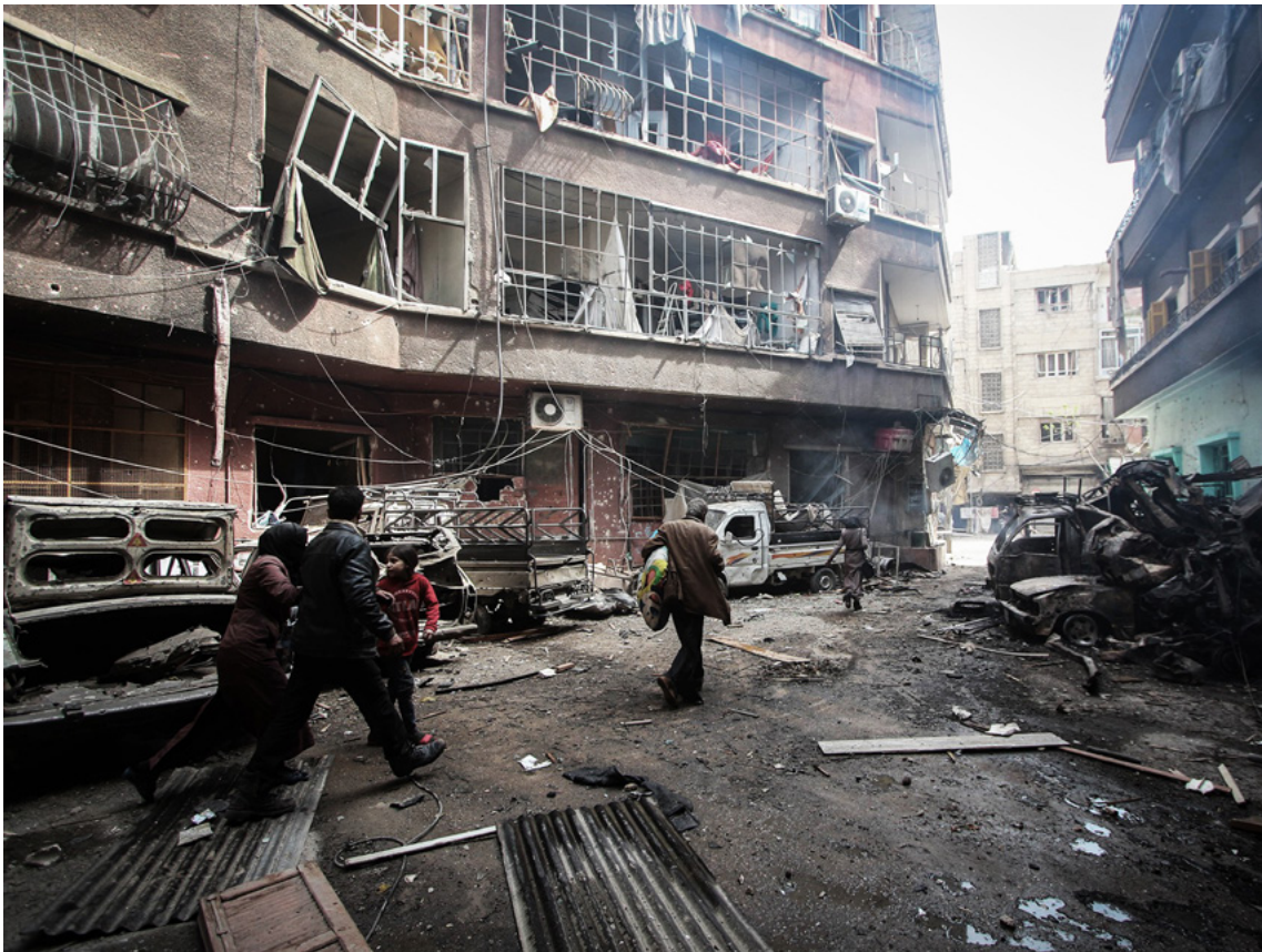
People flee with belongings after their building in Douma was bombed, 20 March 2018. Source: Muhammad al-Najjar
