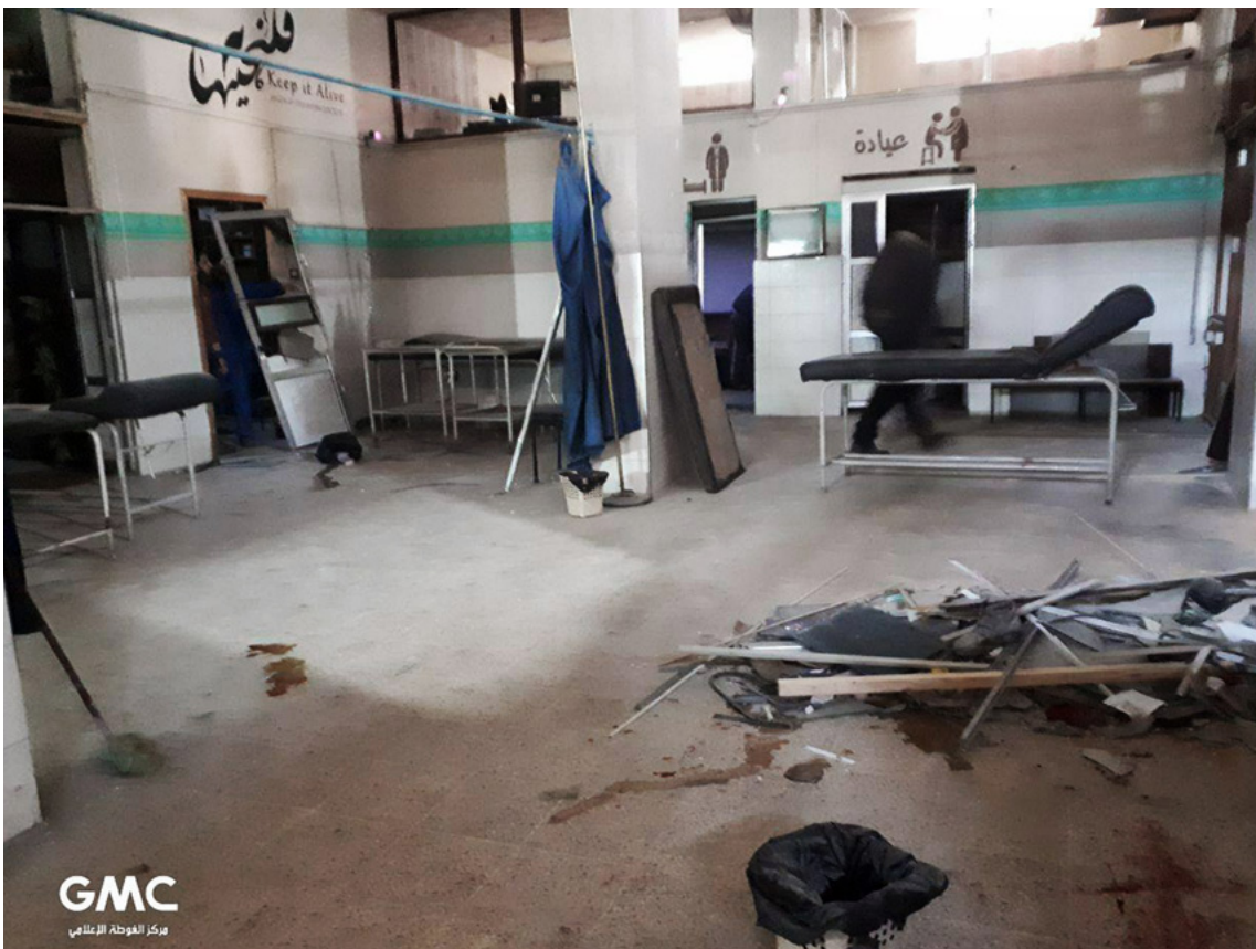
Damaged medical center in Saqba after multiple attacks, 22 February 2018. Source: GMC
