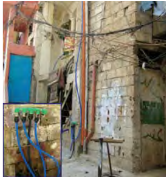
Collective water manifolds recently installed by CISS in Mouhajarin
