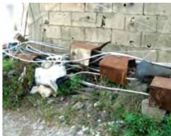
Above-ground water pipes connected by dwellers in Jabal el Halib
