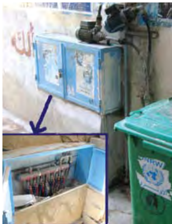
Collective water manifold installed by UNRWA as part of a WATSAN project extended to Mieh Mieh AA
