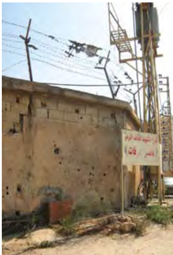
One transformer installed by EDL at the entrance to Tallet el Mankoubin provides electricity to the AA
