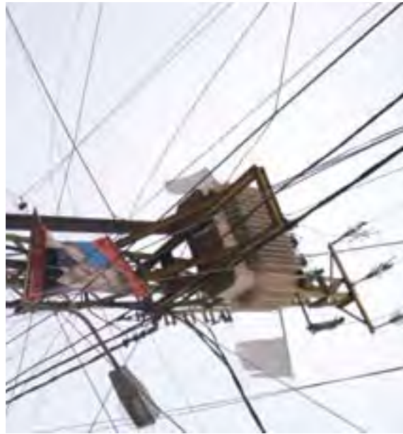
Electricity is provided in Sekke through a transformer installed by the Camp PC using financial contributions collected from dwellers
