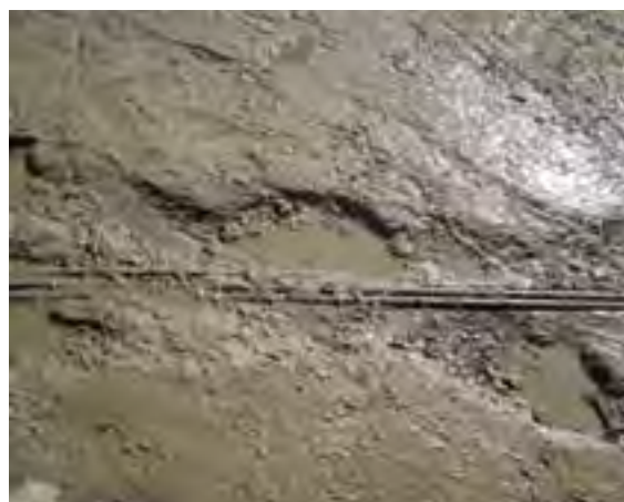
Partially exposed water network in Bustan el Kods
