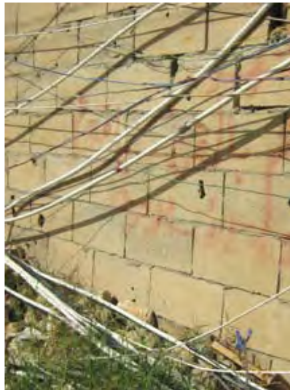
Intertwined electricity and water connections in Jabal el Halib
