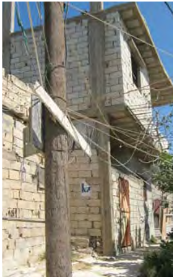
Basic methods for retaining loose and unshielded electricity cables in Hay el Wadi, Mieh Mieh AA
