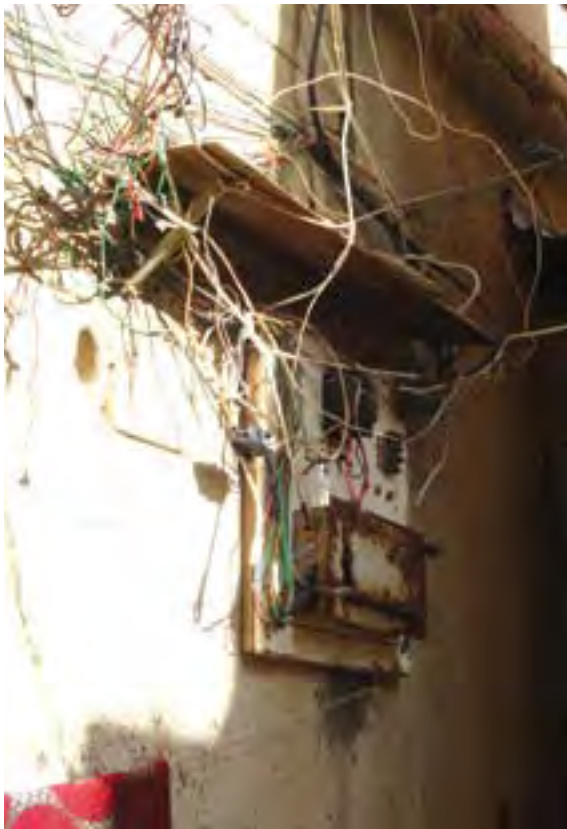
An example of unorganized electricity provision, Bustan el Kods AA around Ain el Helwe Camp
