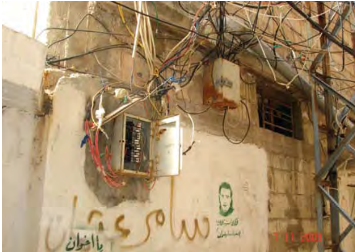
Unorganized connection from the PC/EDL electricity network in Baraksat
