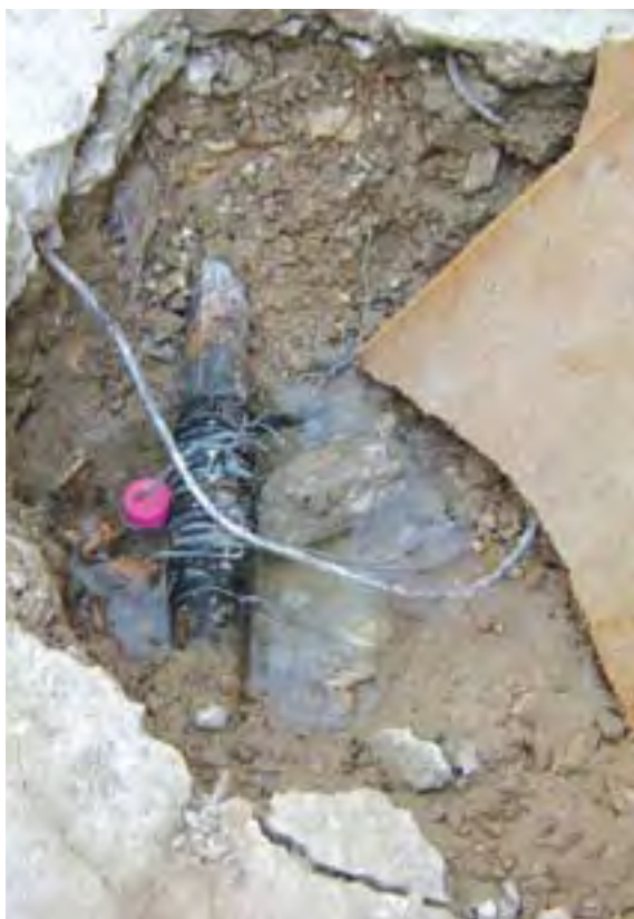
Basic methods of repairing sewage networks, Baraksat AA around Ain el Helwe Camp
