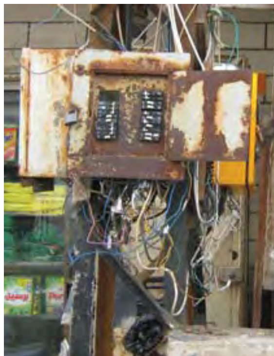
Ad-hoc connections to electric distribution boards, which replaced EDL meters, in Tawari
