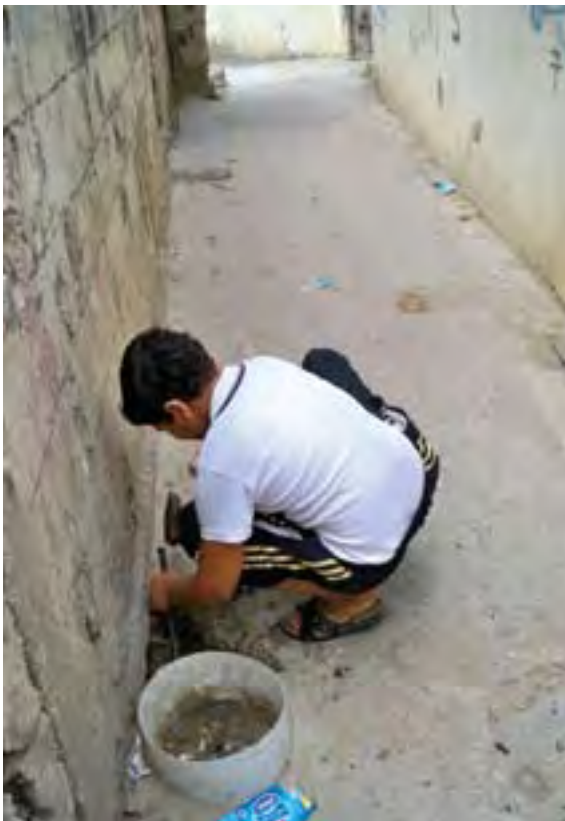
A young dweller resorting to unblocking sewage congestion by manually breaking manholes
