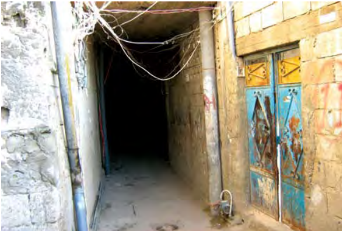
Informal electricity hooking in Bustan about Jamil
