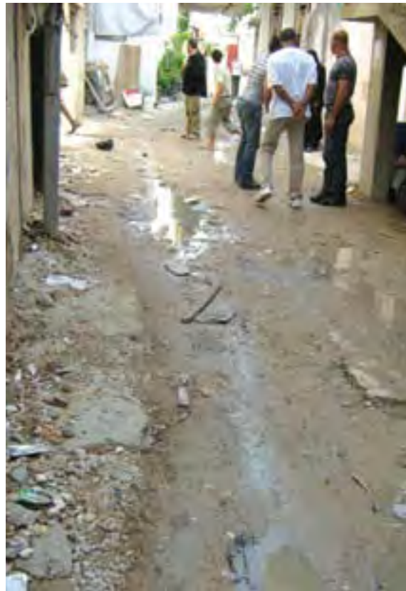
Roads in the AAs are in massive need of rehabilitation and paving, Baraksat AA around Ain el Helwe Camp
