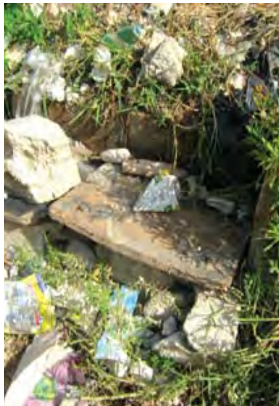
Exposed septic tanks in Jabal el Halib
