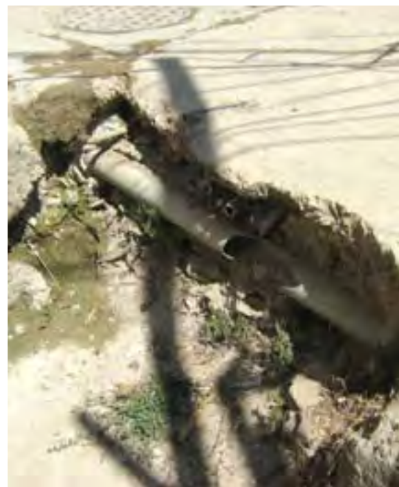
Broken sewage pipes in Mieh Mieh AA
