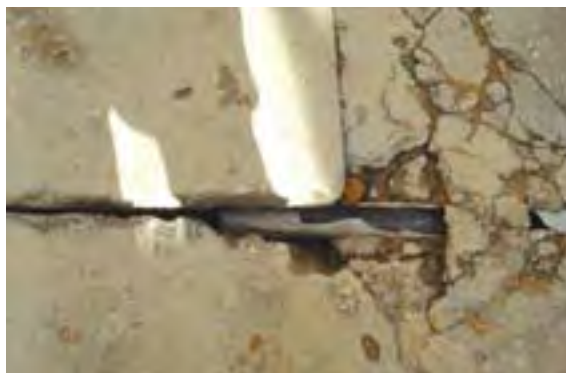
Damaged sewage pipes in Bustan el Kods
