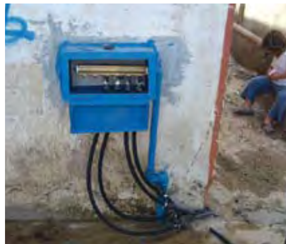
Collective water manifolds installed by UNRWA and UNICEF after the conflict in NBC AA (Source NBRC)
