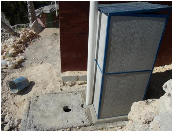
A double pit latrine installed on a steep slope. Each pit is capped by a hand removable slab to facilitate its emptying.
