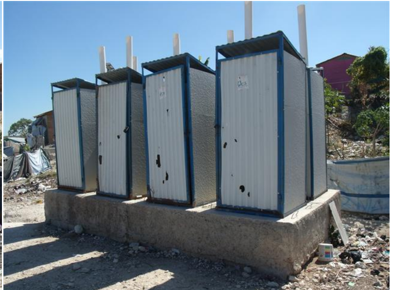
A block of 8 CRS installed vault public latrines in a camp.
