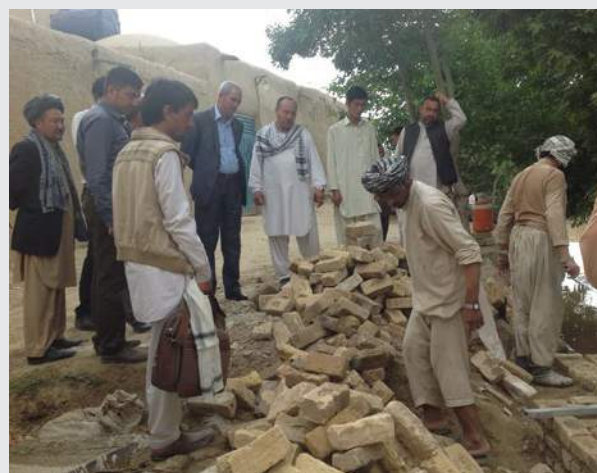
Mazar-i-Sharif MAB Deputy Head monitoring construction progress of CDC sub-project in District 5.
