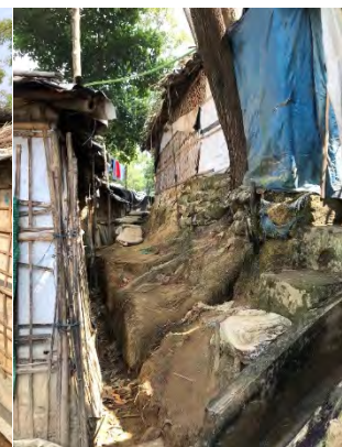
Lack of slope consolidation
