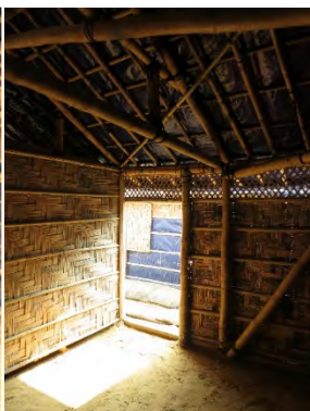
Door & lack of privacy
