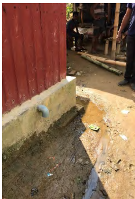
No proper drainage
