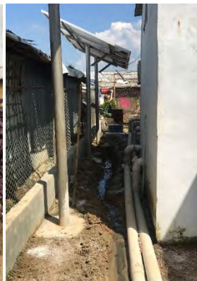
No proper drainage
