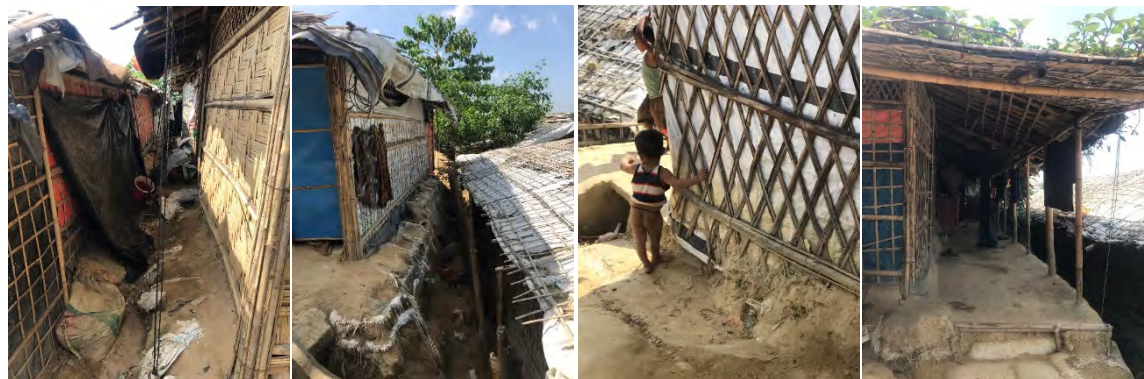
Inadequate drainage and lack of soil consolidation
