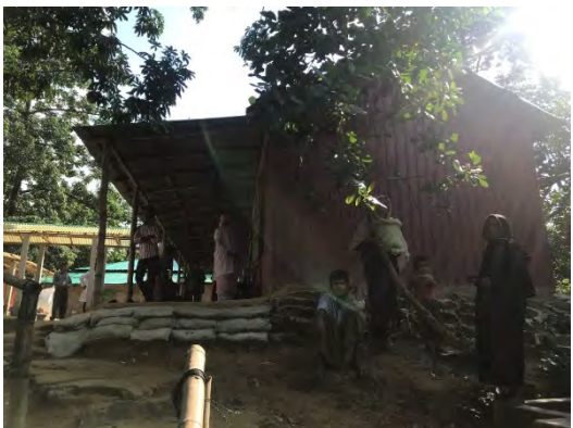
Slope stabilization needed (front side)
