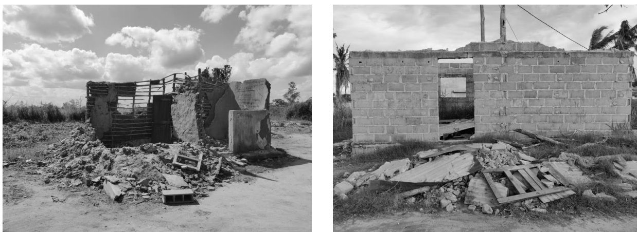
Pic. 2. Common damages to traditional and conventional houses.
