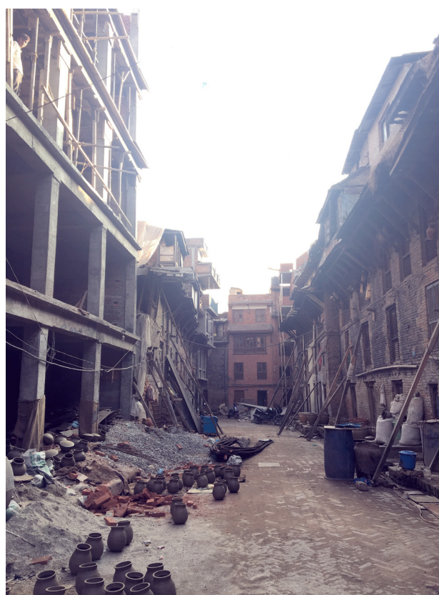
Thimi, February 2017: on the left a new RC frame structure is being constructed while on either side traditional houses have timber props providing support from the street.
