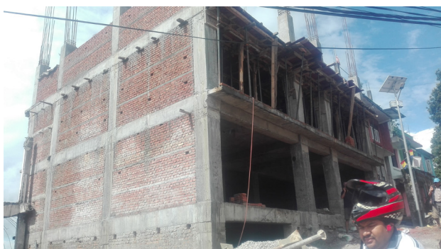
Housing Typology: Reinforced Cement Concrete Framed Building (RCC) Location: Sindhupalchowk, Chautara Municipality The house owner has received the second tranche of the GoN housing reconstruction grant.
