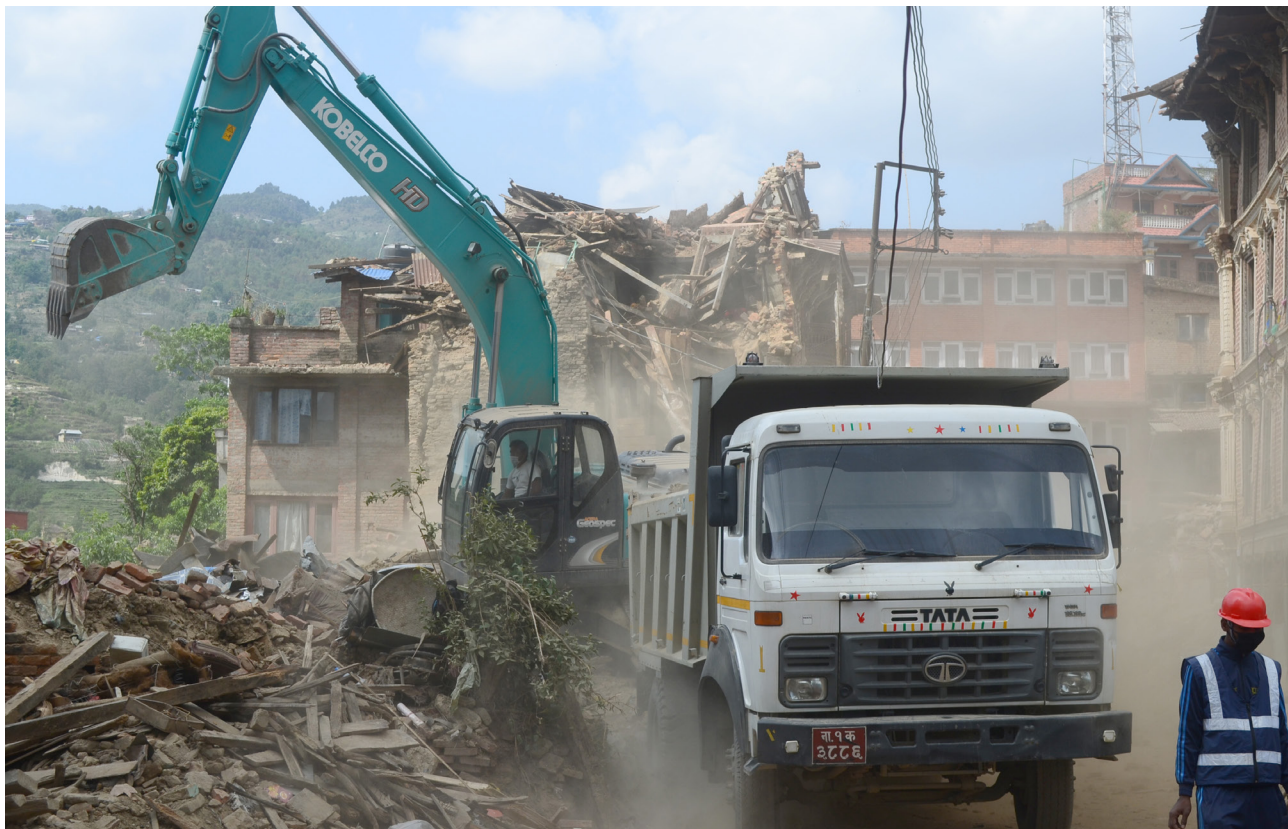
Demolition being carried out by the Nepal Army in Sankhu, Shankharapur Municipality, Kathmandu on 20 May 2015.
