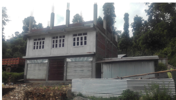
Housing Typology: Reinforced Cement Concrete Framed Building (RCC) Location: Sindhupalchowk, Chautara Municipality The house owner has received the second tranche of the GoN housing reconstruction grant.
