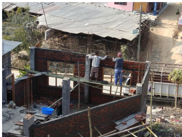
Housing Typology: Reinforced Cement Concrete Framed Building (RCC) Location: Ramechhap, Manthali Municipality, Ward No. 1 Irregular shaped RCC house with columns that are 9"x 12".
