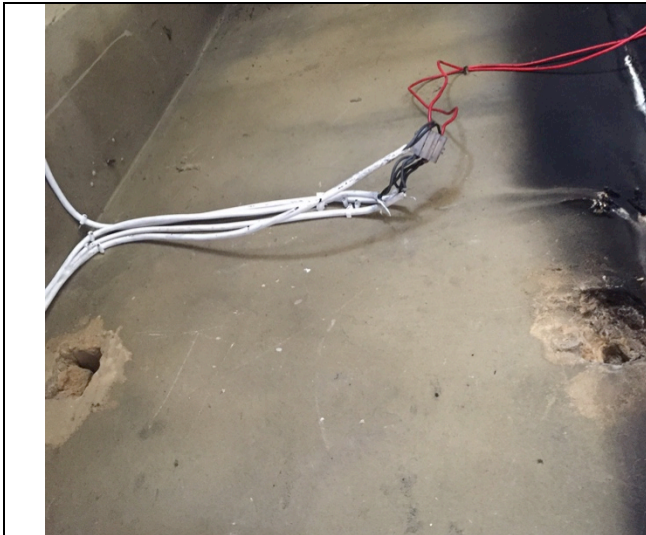
Abu Samra: Electric cables
